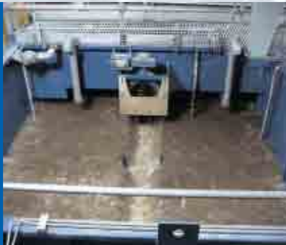
Backwash water flowing in trough, air assisted.
