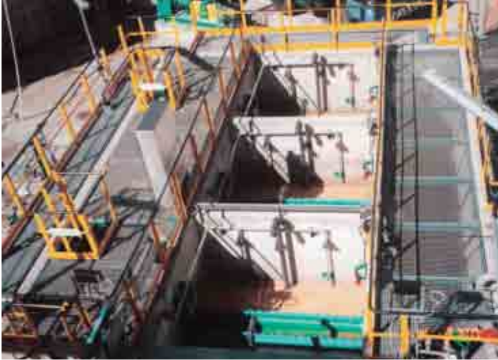
The Hydro-Clear® sand filtration system filters secondary effluent for a wide variety of applications, including refinery wastewaters.
