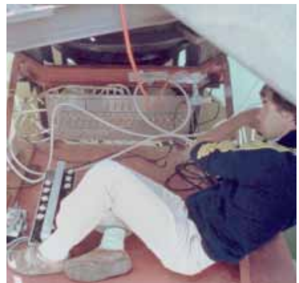
Installation of sample probes in header.
